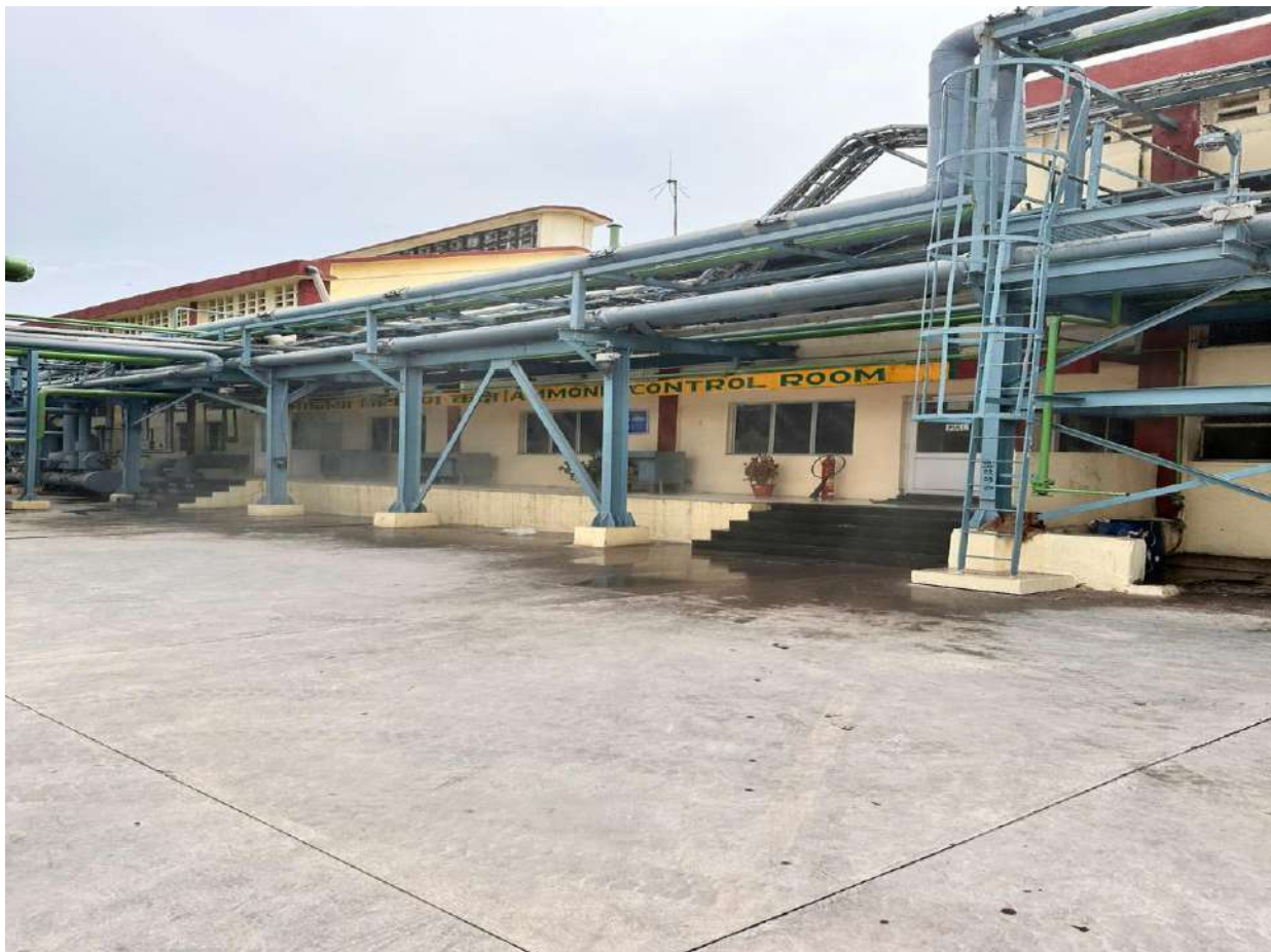
Water curtain system started outside Ammonia Control Room
