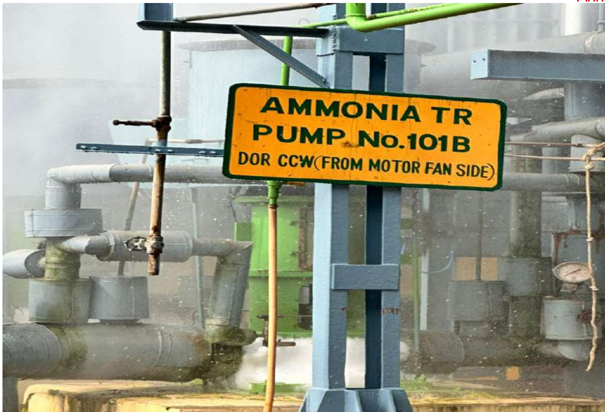
Water Sprinkler system started at Ammonia Tank B.
