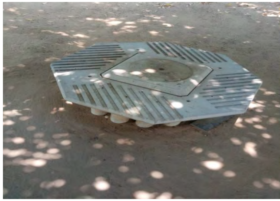
Module installed near Sr. GM Bungalow
