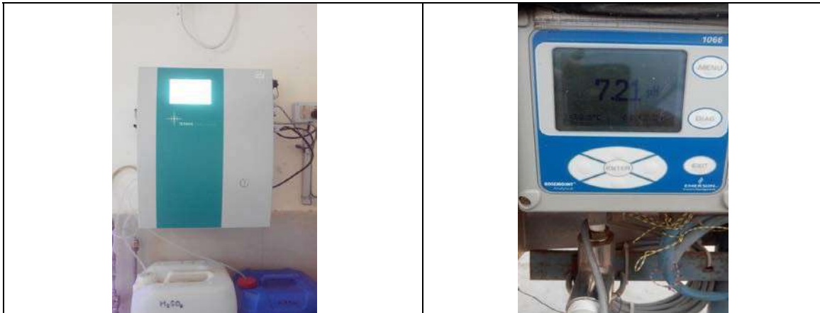
Online Ammonia Analyzer at ETP
