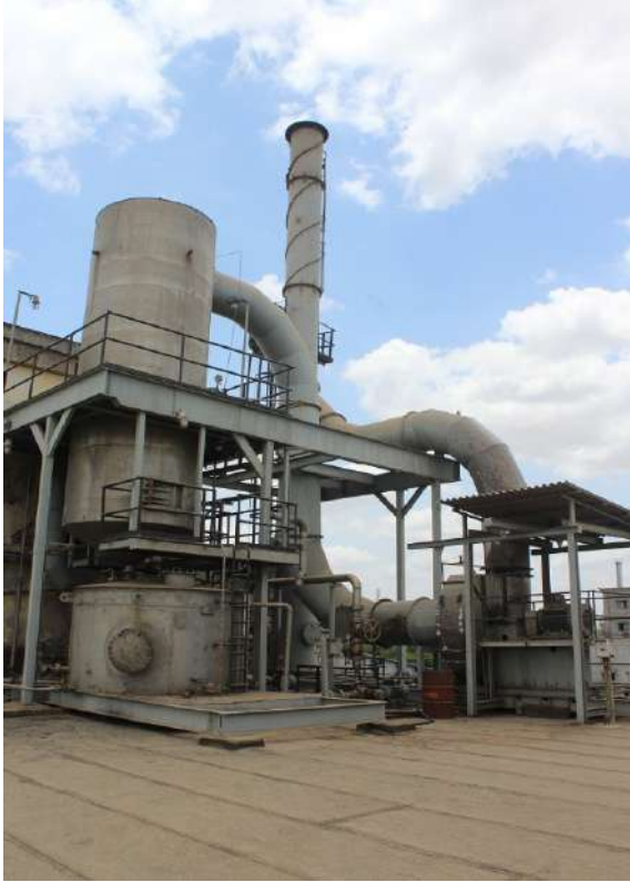
Dust Extraction System in Bagging & Product Handling Unit
