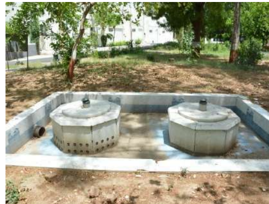
Rain Water Harvesting system (New) (25 m 3 /hr capacity)
