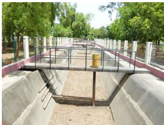
Rain Water Harvesting system (Old) (36 m 3 /hr capacity)
