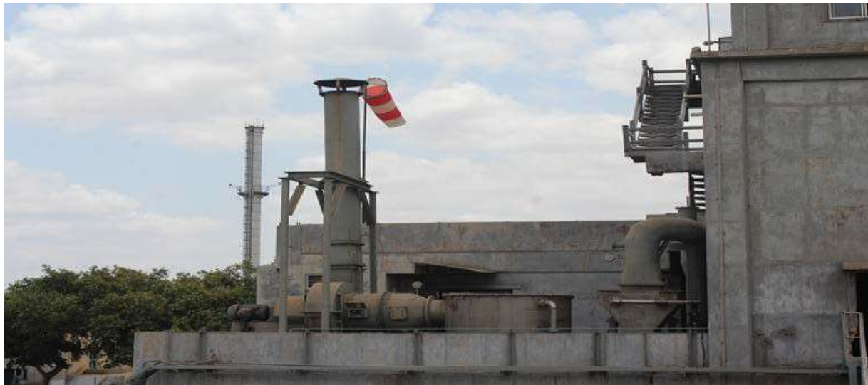
Dust Extraction System in Silo (Urea Storage Area)
