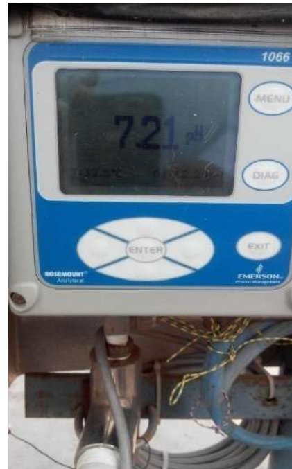
Online PH meter at ETP
