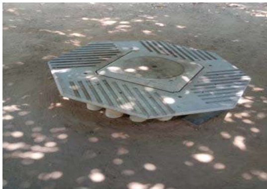
Module installed near Sr. GM Bunglow
