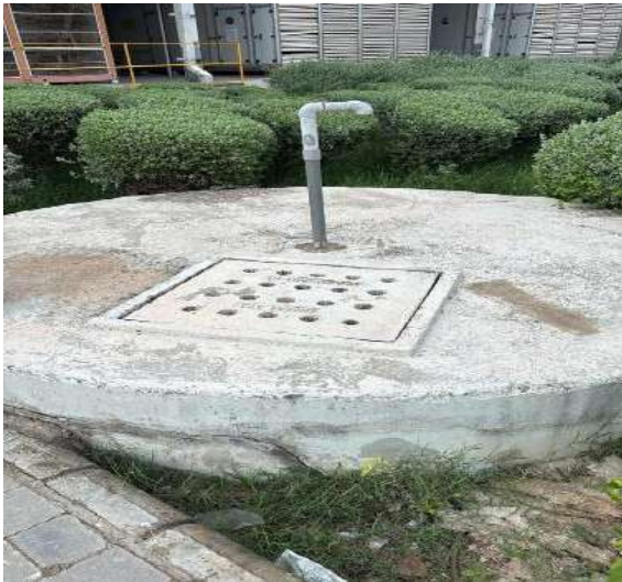
(Recharge well near Reynold Chiller1)
